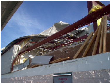
Charlotte County, Florida: County EOC damaged and emergency generators flooded in Hurricane Charley
